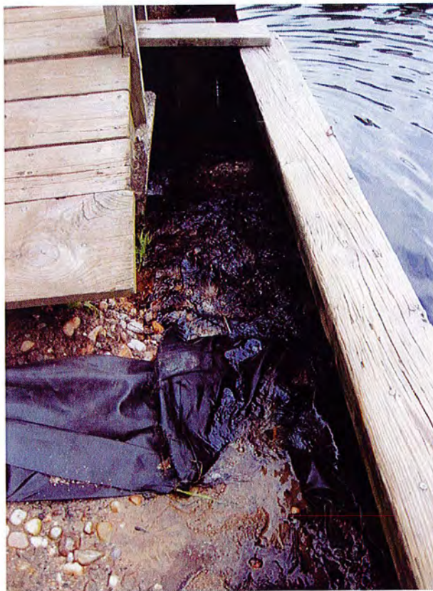
Photo # 2: Seepage through wooden bulkhead
